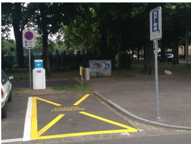
Abbildung 6: General Guisan-Strasse, 22 kW
