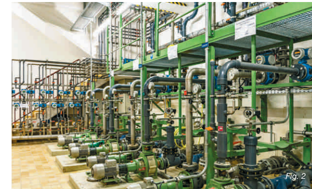
Pump cellar of the Rhine monitoring station
